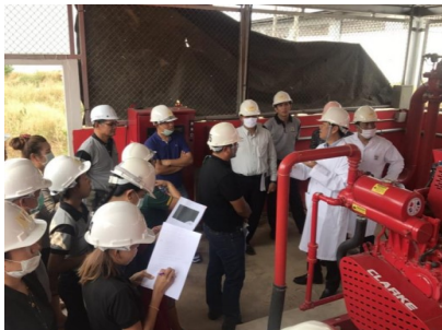
The inspection of the Fire Suppression System (Phu Kham Animal Feed Plant in Laos)
